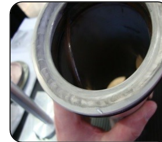
Spring detected in filling indicator of the main gear
