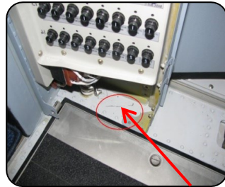
Wire in fuse box
