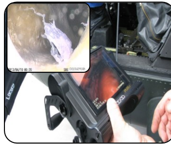
Material delamination inside helicopter ventilation channel
